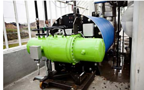
Energy From Waste Pyrolysis Plant
